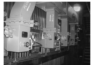
New side wall OFA was installed on this combination waste wood and oil fired power boiler.
